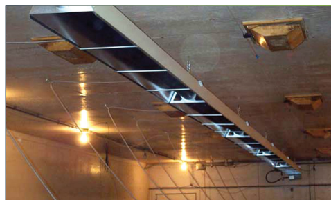
Figure 4. Typical infrared heater Source: Prairie Swine Centre
